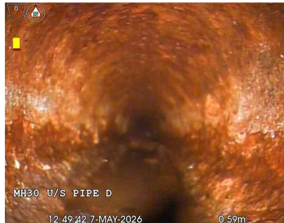
2, 00:00:12, 0.59 m Attached deposits, other from 12 o'clock to 12 o'clock, 5% cross-sectional area loss, start, Rust build up
