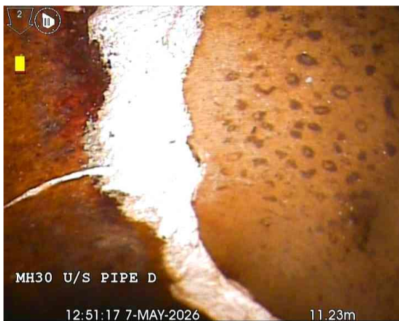
3, 00:01:47, 11.24 m Crack, circumferential from 7 o'clock to 9 o'clock
