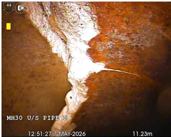
5, 00:01:57, 11.24 m Crack, circumferential from 3 o'clock to 5 o'clock
