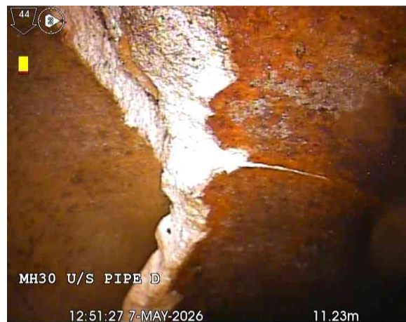
4, 00:01:57, 11.24 m Attached deposits, encrustation from 9 o'clock to 3 o'clock, 5% cross-sectional area loss
