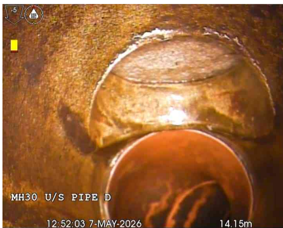
7, 00:02:33, 14.15 m Junction, closed at 12 o'clock, 150mm dia
