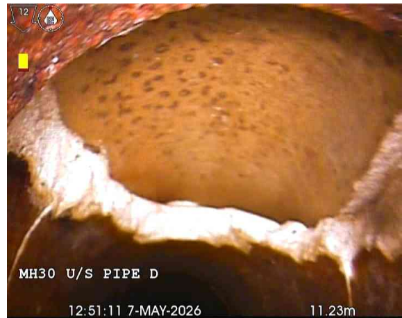
6, 00:01:41, 12.40 m Defective repair, separation from host pipe from 11 o'clock to 1 o'clock, Hole covered by pipe piece. not properly sealed
